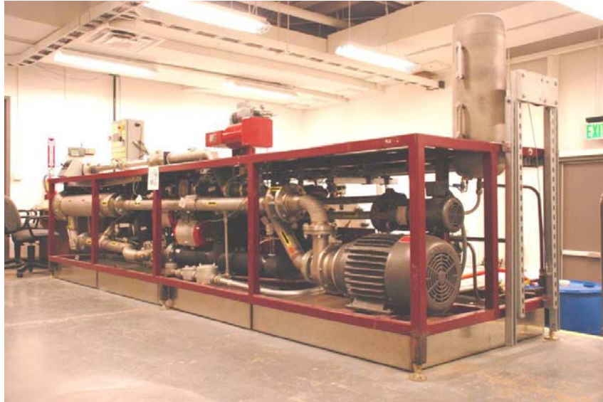
Figure 8. Flowmeter Calibration Setup
